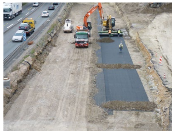
Bridging of sinkhole (Bochumer Westkreuz motorway interchange [A 52], Germany)
